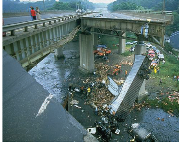
Mianus River Bridge, Connecticut, 1983 rust formation and fatigue cracks
