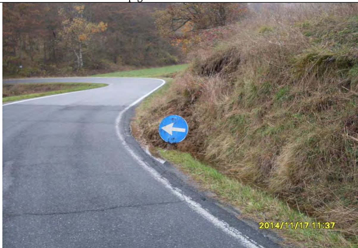
SP 215 "Spigno-Pareto" km 6+380 sx n°1
